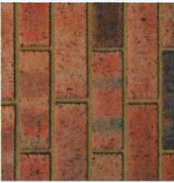
TYPE EX1 Red brick in a stretcher bond pattern. IBSTOCK Wylam Olde Blend or similar approved.
