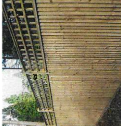
TYPE B3 1.8m high close timber boarded timber panels with trellis top or similar approved.
