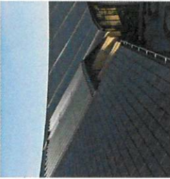
TYPE R1 Artificial slate roof tiles by Marley Eternit - Rivendale Fibre Cement - colour blue black or similar approved.
